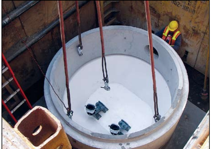
Contractor George Schmid & Sons has installed many Romtec Utilities pump stations in the Camas, Wash. area.
