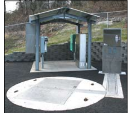
New wet well and control shelter.
