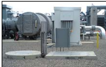
L-R: wet well w/pump disconnect panel, valve vault, control panel (back of panel visible)
