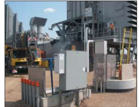
Open for business - second pump station pictured during start up and testing.
