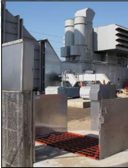
Pump station (foreground) and generator.
