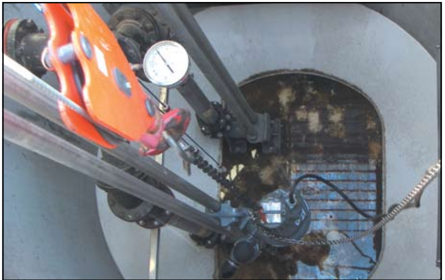
ITT Flygt submersible pump lowered into wet well.
