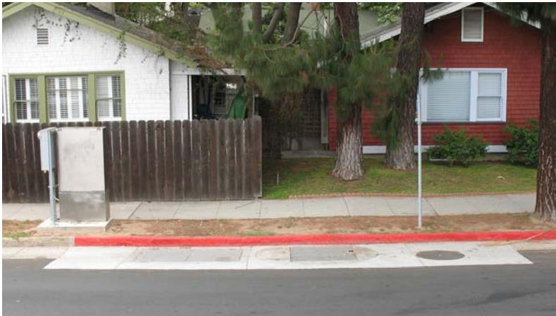
Haley Street lift station is constructed at grade in traffic lane.
