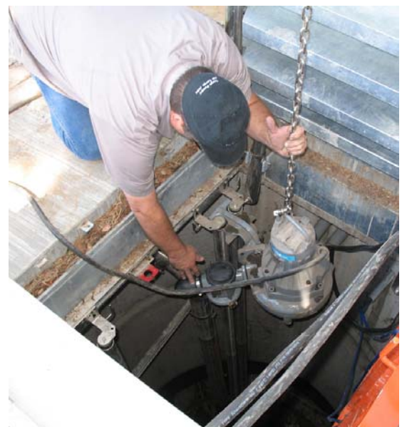
ITT Flygt submersible pump with mix/flush valve is installed.
