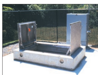
Finished lift station site has top slab with standard aluminum hatch doors.
