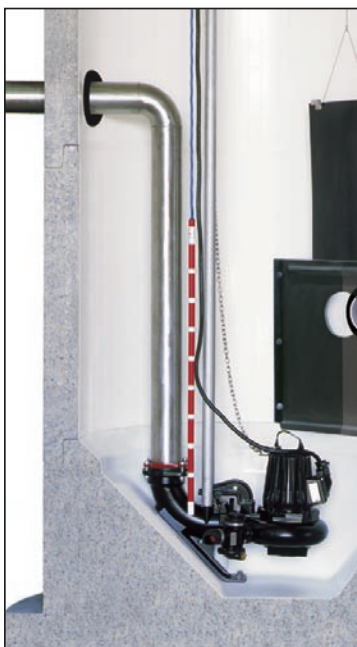
This section view shows the MultiTrode liquid level sensing probe suspended in the wet well.
