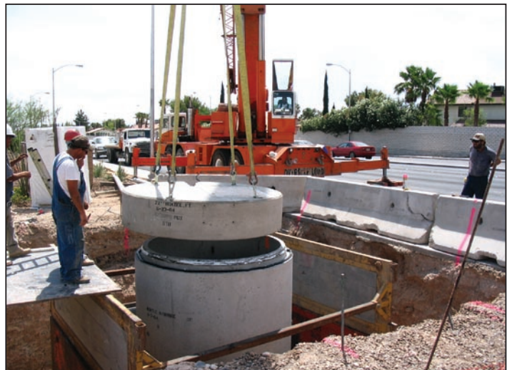
A crane places the top slab to finish off the wet well installation; the base, barrel and top slab are all pre-aligned for ease of installation.
