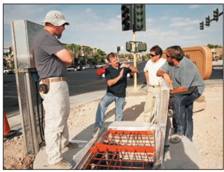
Romtec Utilities' Jim Baird explains to contractors how the deflector panel governs flow; top slab is shown with the hatch door open and the safety grate visible.
