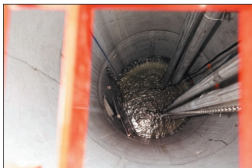
The wet well fills with water after start-up; the storm pipe is visible in the well wall to the left.
