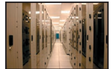
The MultiTrode-managed infrastructure offers reliable and secure servers that are monitored 24 hours a day.
