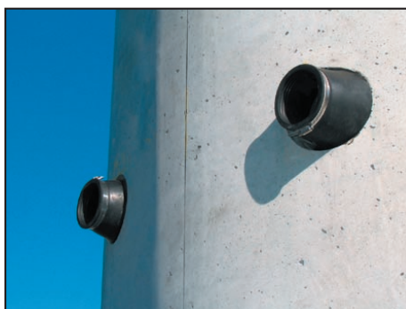
A Kor-N-Seal flexible seal is fitted into each wet well penetration to accept the influent and discharge pipes.
