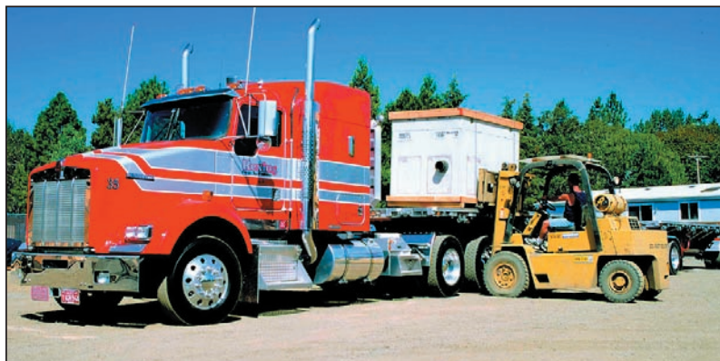
The pre-cast concrete valve vault arrives at the job site ready for installation.
