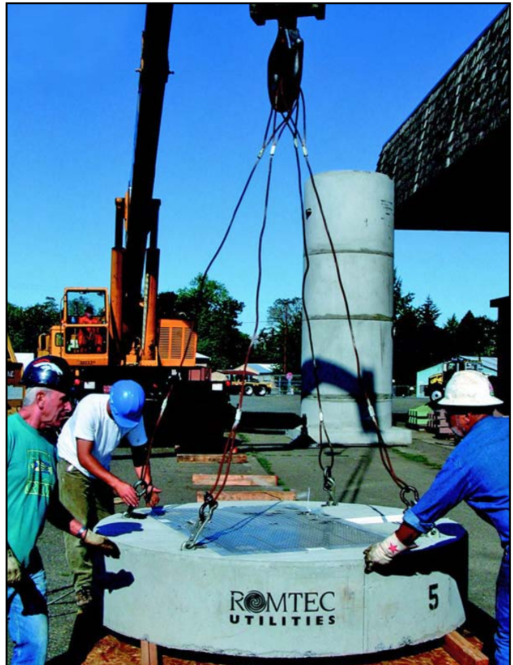
Romtec Utilities workers prepare to stack the pre-cast top slab before painting alignment marks on the barrel sections.
