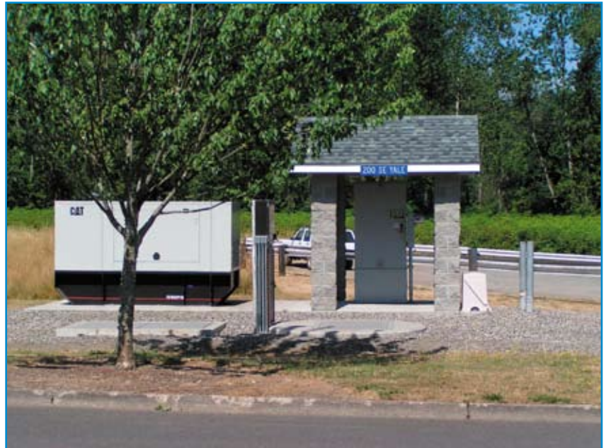
Two finished wet well sites at Camas, Wash. Above, the One-Stop lift station, with a shelter building protecting the control panel, and below, the Larkspur station.
