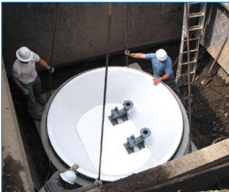
Workers carefully align the precast wet well base at Echo Glen Children’s Center.
