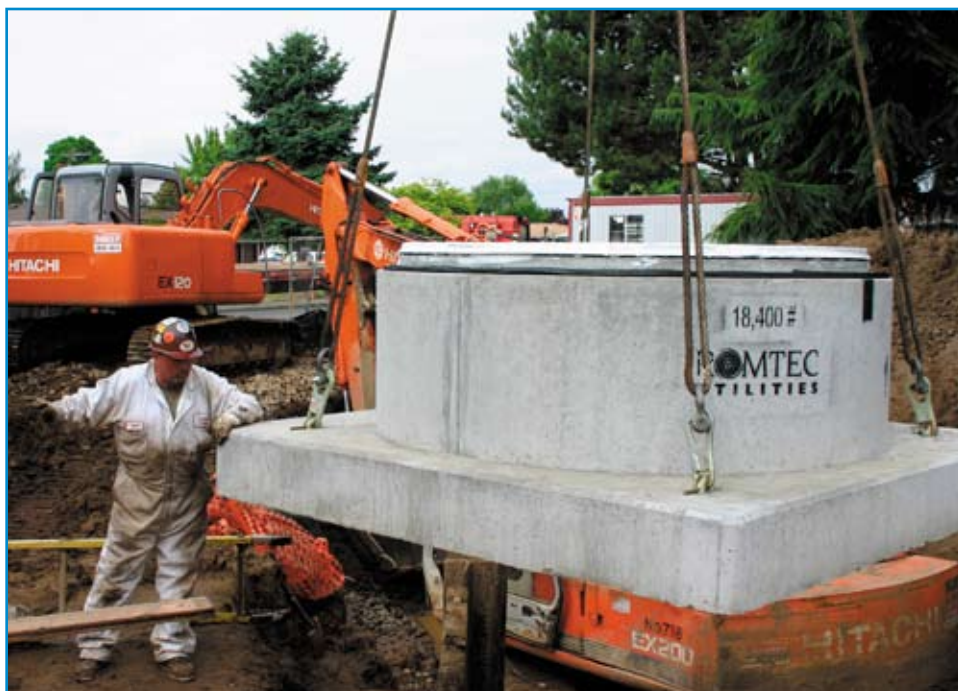
Expert delivery and installation are a key part of every Romtec Utilities lift station. Here, a wet well base is installed at Woodburn, Ore.
