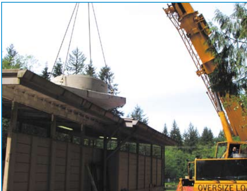
The crane palcing the concrete wet well starts by lifting the 17-ton precast base over a small building.
