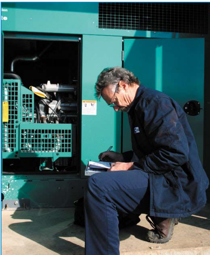
A Cummins Northwest technician records data from the on-site generator.
