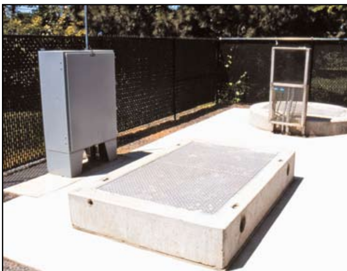
Electrical and communication systems are often subject to complex municipal standards that are most efficiently dealt with during the lift station's design phase. At top, an enclosed the Cummins standby generator is housed in a QuietSite II sound-attenuation closure, a common standard in many municipalities. It is also common to find guidelines for the look of a finished submersible lift station site, at bottom.
