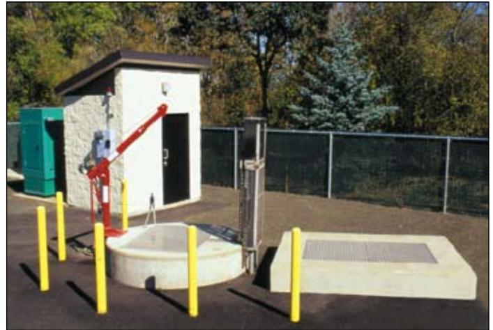
SplitLok 6'-8" x 8'-8" concrete building: electricals are inside, disconnect panel and power meter outside.
