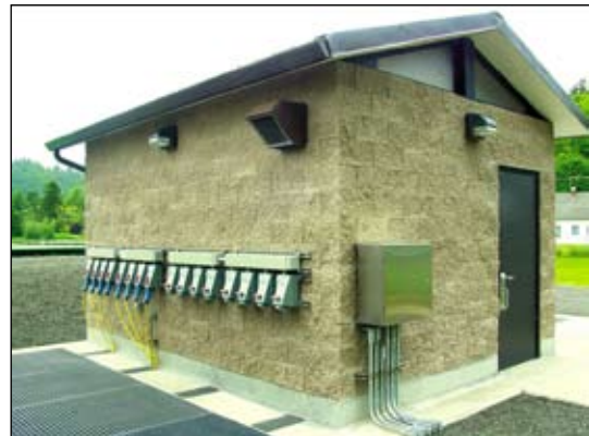
Mid-size control building with multiple penetrations, triple disconnect panel outside.
