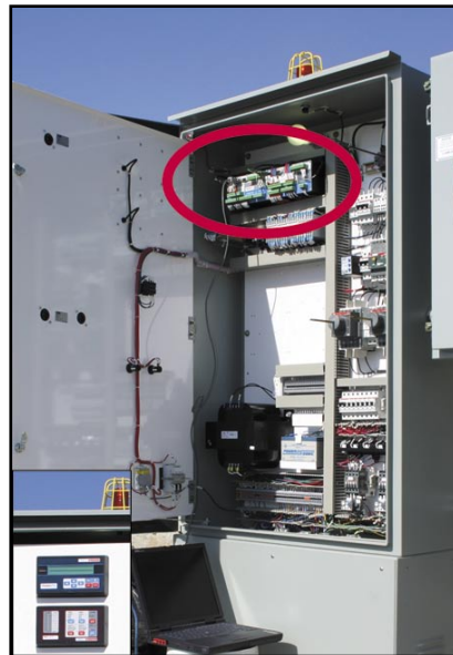
The open dead front of a Romtec Utilities control panel reveals components of the MultiTrode MT2PC Pump Controller and MonitorPro Pump Station Supervisor, circled items and inset photo. The Flygt technician's computer, at bottom, is used for programming and testing during lift station start up.
