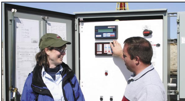
Kelly Wood, OTAK project engineer, left, and Andy Dake, Romtec Utilities technical sales, discuss the MultiTrode components in the lift station at Hillshire subdivision in Camas, Wash., a project of Centex Homes.
