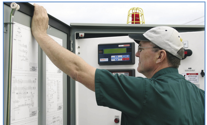
Tim Curns, ITT Flygt Field Technician, reviews the detailed control panel drawings of a Romtec Utilities panel equipped with MultiTrode's MonitorPro.
