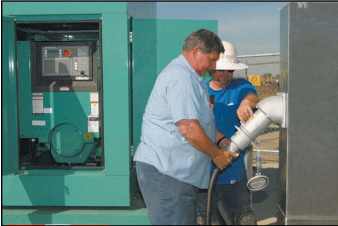
Anderson Pacific electrician Rick Melena, left, and Cummins technician Richard Zwaal test connection of the generator power cable to the control panel receptacle at the Line M stormwater lift station in Union City, Calif.
