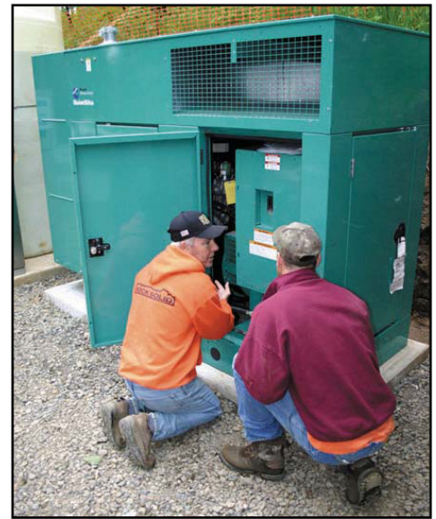
Workers from George Schmid & Sons inspect the Cummins generator housed in a QuietSite II sound-attenuation enclosure at the lift station site for the Cassini View subdivision in Ridgefield Wash.
