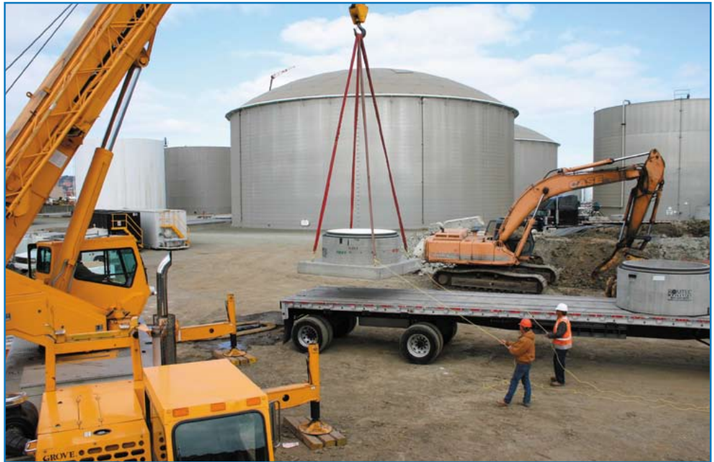
A crane is used to unload and place precast concrete wet well base.
