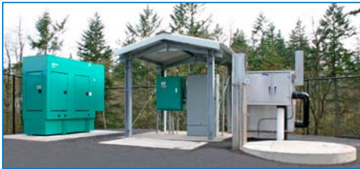
A steel shelter protects the control panel and generator transfer switch at the Hunter Ridge lift station in Camas, Wash. City public works officials have decided to integrate this structure into all of their lift station layouts, in order to protect electrical components from temperature extremes and provide maintenance workers with a covered area.
