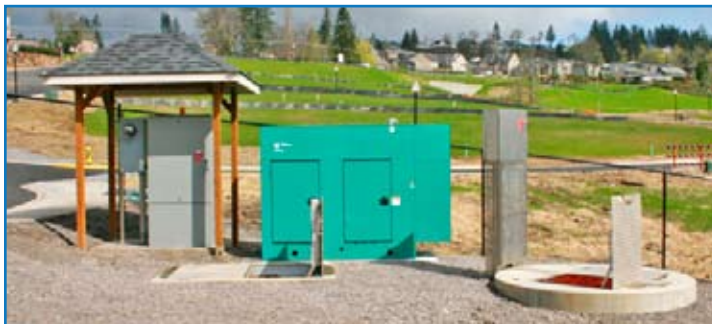
Daniel Park in Washougal, Wash., efficiently uses a small footprint to fit all of the lift station components, including, from left, a shelter of City of Washougal design, pre-assembled valve vault, enclosed Cummins generator, and wet well with duplex Flygt submersible pumps and disconnect panel.
