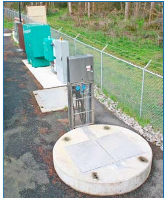
The Larkspur lift station in Camas, Wash., features a distinctive linear layout, with all components lined up in a space-saving row.
